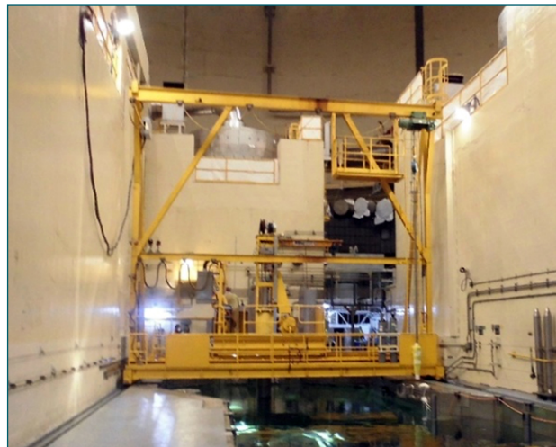
Figure 5. Containment fuel manipulator crane overview.
