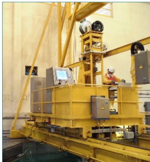
Figure 6. Containment manipulator trolley and equipment.
