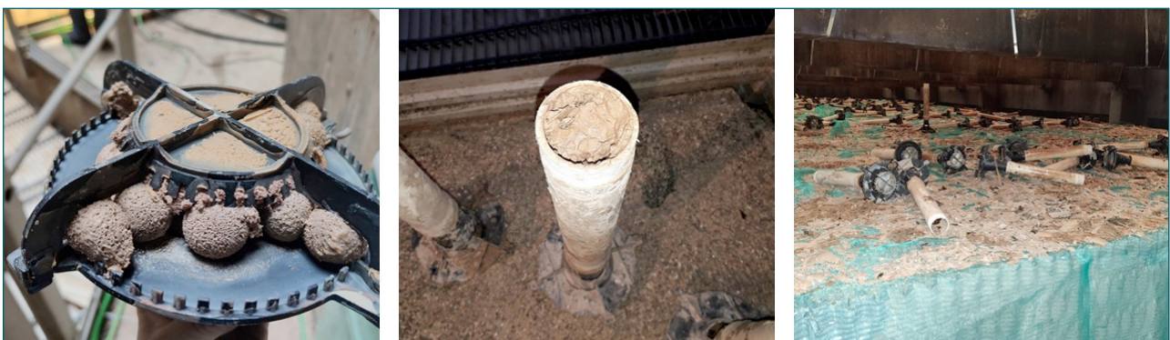
Figure 6. Preliminary condition of nozzles.
