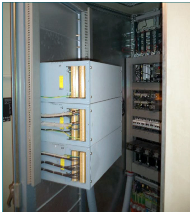
Figure 4. Existing excitation system and synchronization (in swing frame) in existing cabinet.
