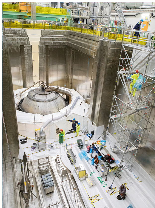
The top of the reactortank of Ringhals 1. © Photo Ringhals.
