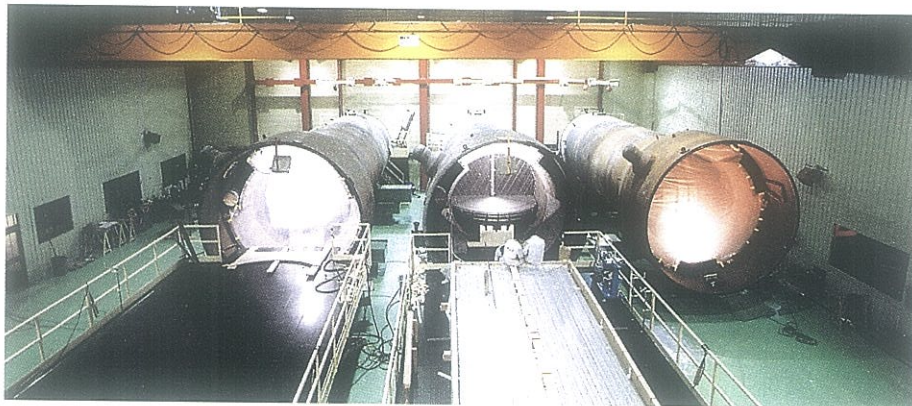
Steam Generators for Doel - 3 in clean condition room.
