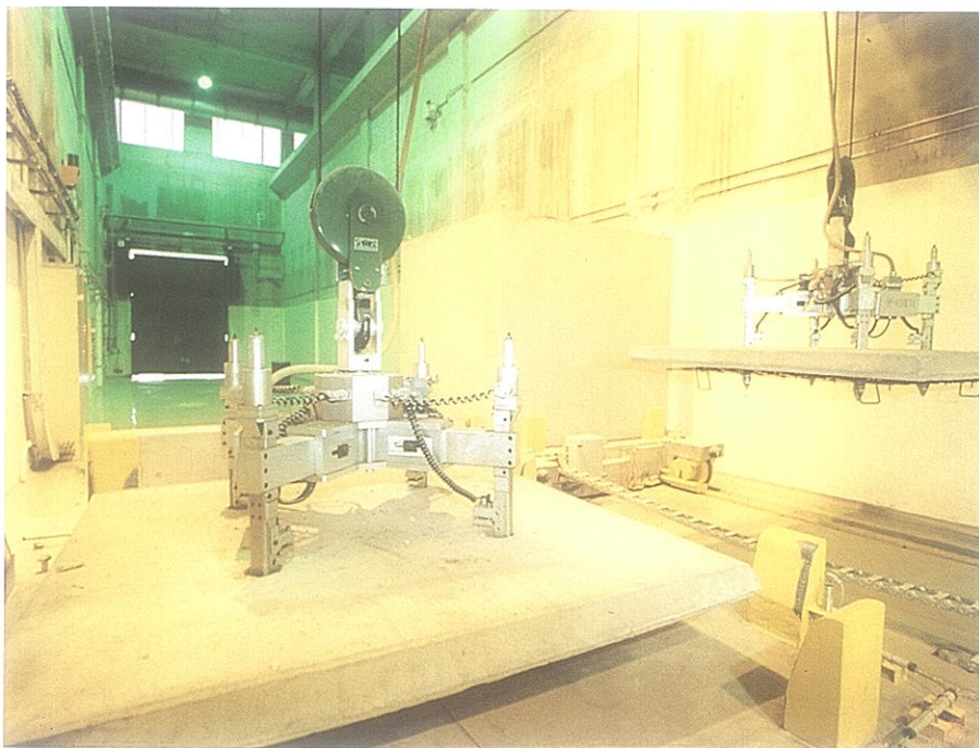
Gripper of the bridge crane in the compacting building.
