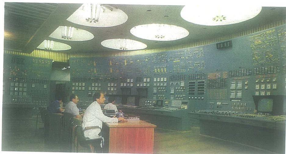
Unit 2 control room
