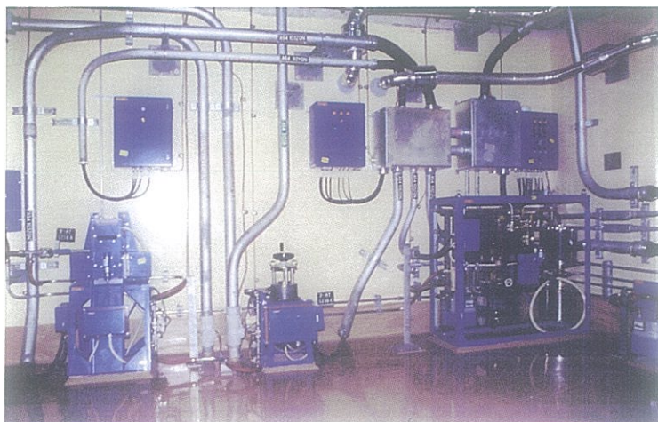
Discharge pipe monitoring
