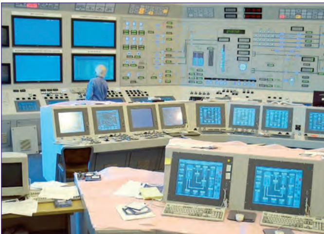
Sala de control de la central de Lungmen. Lungmen Power Plant Control Room.
