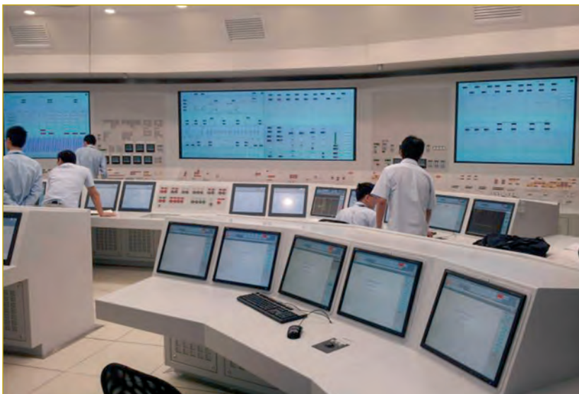
Figura 5. Sala control de Fangjiashan, CPR1000 (Cortesía CNPE).
