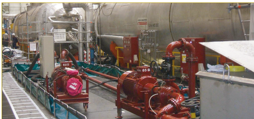
MSR and chemical impulsion area.
