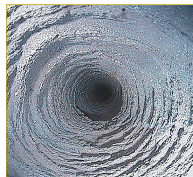
Interior of MSR pipe with magnetite deposits.
